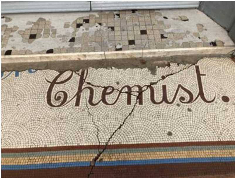
Figure 24: Damaged mosaic threshold at Broadway Mansions
